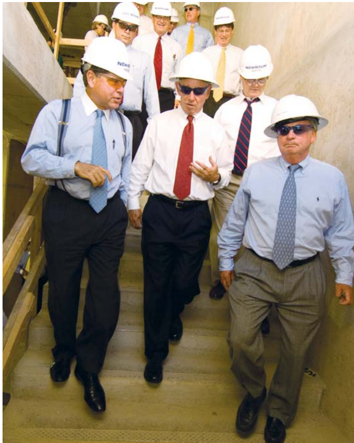
Newseum Chairman Alberto Ibarguen, left, confers with Charles L. Overby, center, and Peter Prichard as they lead trustees on a tour of the construction site on Pennsylvania Avenue.
